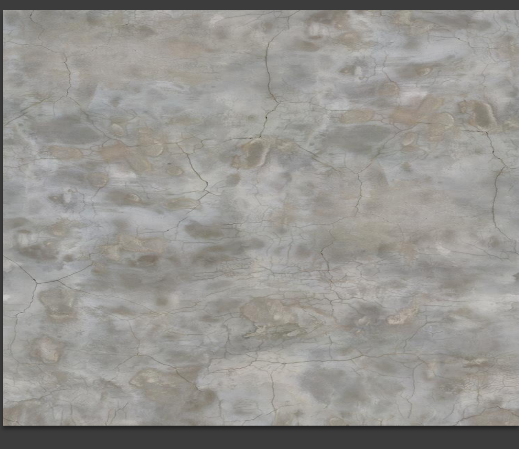
Concrete texture FCC 025 Cracked concrete
